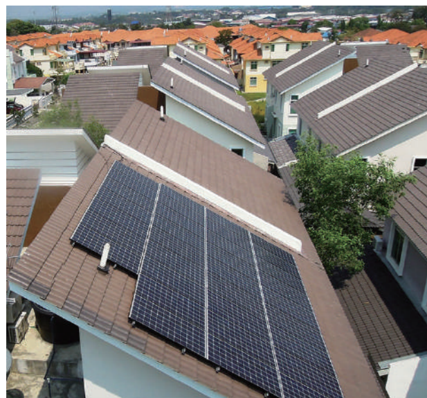
Residential Project in Malaysia 3kW
