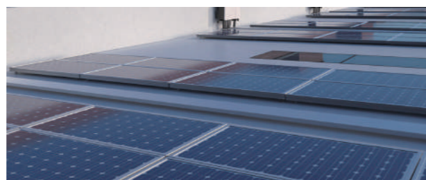
Residential Project in Poland 3kW
