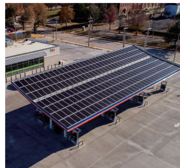
Gas Station Project in Brazil 26kW
