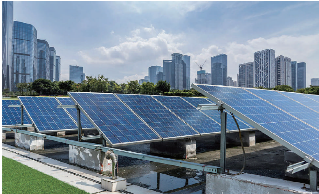
Residential Project in Sweden 10kW
