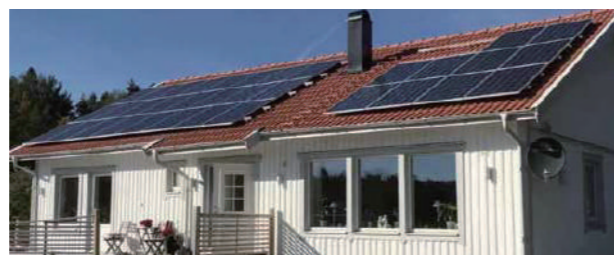
Residential Project in Sweden 10kW
