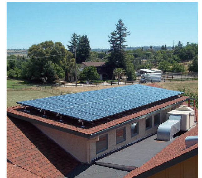
Residential Project in Mexico 5kW
