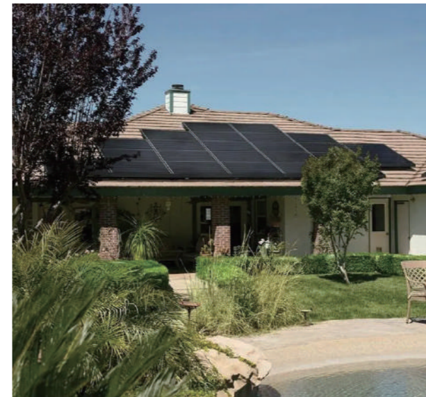
Residential Project in USA 10kW
